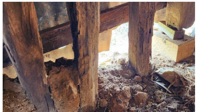
Before conservation, the footings were rotting away. Thanks to supporters like you, they will now keep the cottage standing.
