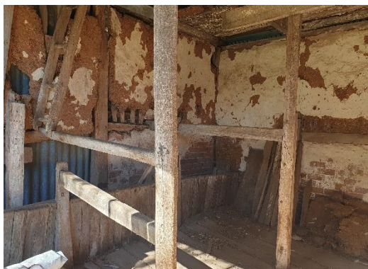
The interior wall of the stable still has large areas of limewash remaining.
