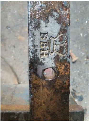
An original gutter bracket
