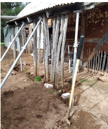
The verandah posts were hanging like windchimes.
