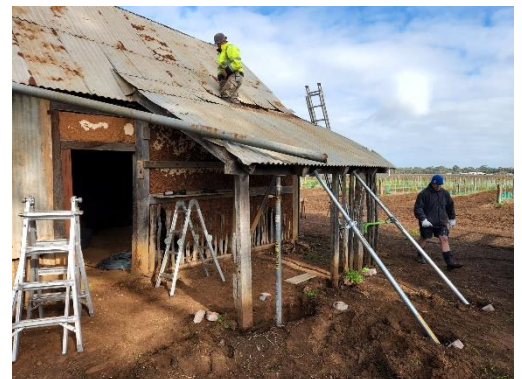
The verandah needed re-aligning
